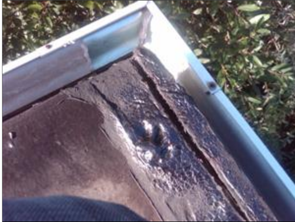
Open joint at roof level
