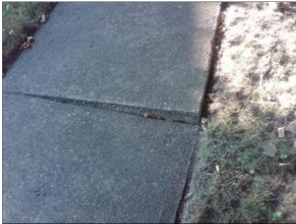
Typical Trip hazards
