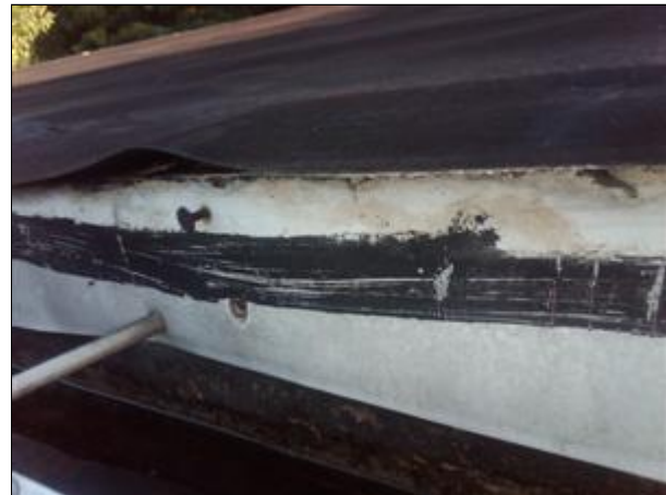
Open joint at edge
