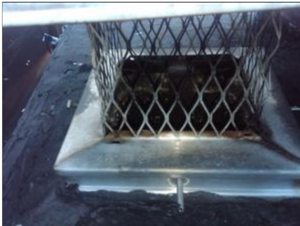
Age and wear noted on flue
