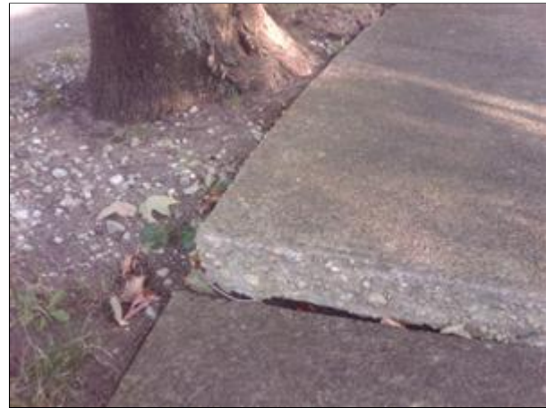
Typical Trip Hazard
